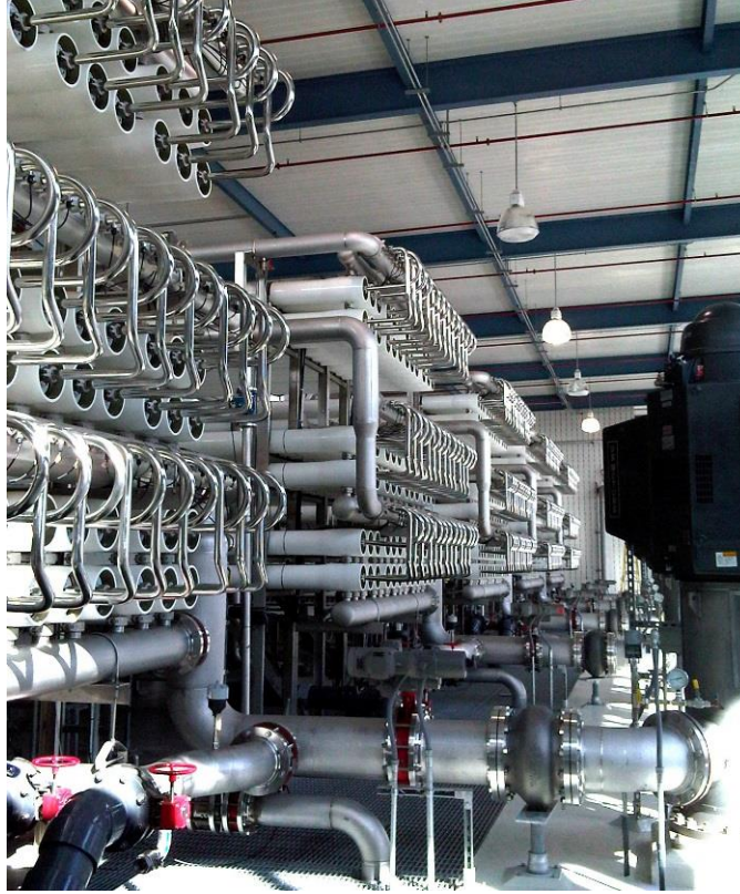
Figure F-2. Photograph of reverse osmosis system.
